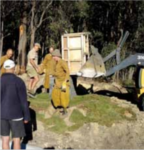
Installing the volcanic name stone from Indonesia, carved from the same volcanic stone as that used for Borobudur, at Jhana Grove
